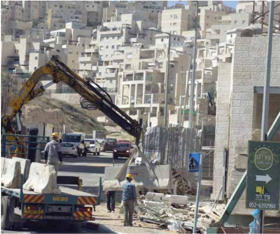
Labourers work at a housing construction site in the Israeli settlement of Har Homa in east Jerusalem on 27 February 2013. The EU has urged its members to block funding for any settlement activities.
